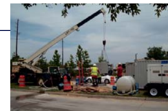
Lowering the MTBM into the tunnel shaft, in preparation of installing 12" clay pipe – in the Industriplex Area.
