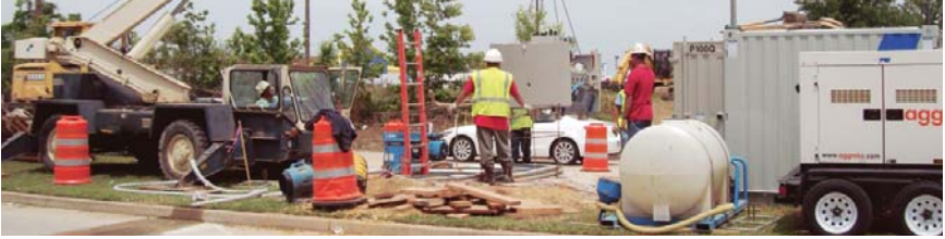
The microtunneling boring machine is lowered into the tunnel shaft at the Industriplex Area project.
