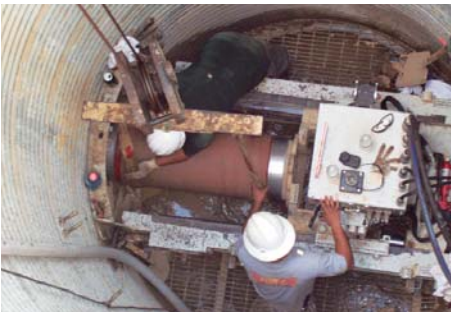
The microtunneling bore machine pushes through a 12 foot diameter heavy-wall clay pipe.
