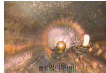
Approximately 238,425 linear feet of pipe was inspected in the Oak Villa area.
