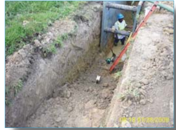
Trench boxes are used for the gravity line installation in the Comite – Foster Area.
