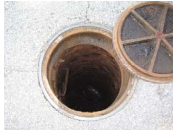
Manhole inspections provide insight into pipeline conditions in the Sharp Road - Florida Blvd. project.
