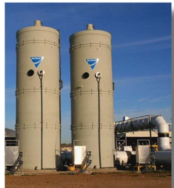
Typical bio-tower installation.
