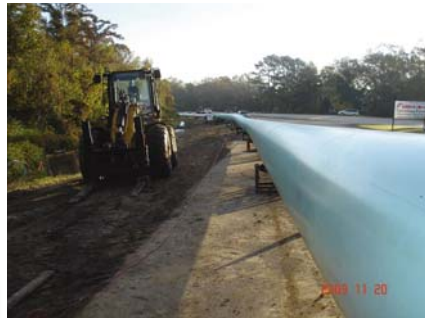
A 12,000' foot long, 36" diameter fusible PVC pipe is being installed along Hooper Road.
