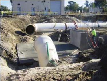
Construction of yard pipe at the SWWTP that will convey wastewater throughout the Plant.
