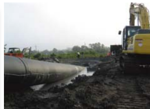
The entry pit for the 65" HDPE pipe is installed using the HDD method.
